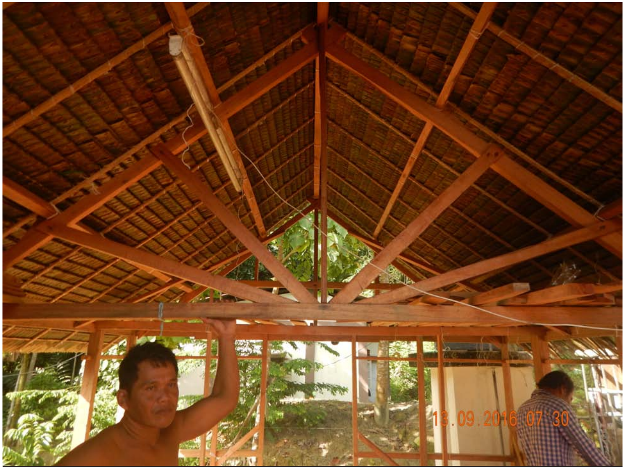
Figure 2. New thatch roof made with Nypa fruticans at Pulo Panja village, Little Nicobar Island.
