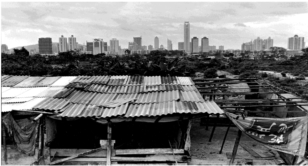
Figure 2.6 The demolition of Pearl River Village at the core area of the PRNT.
