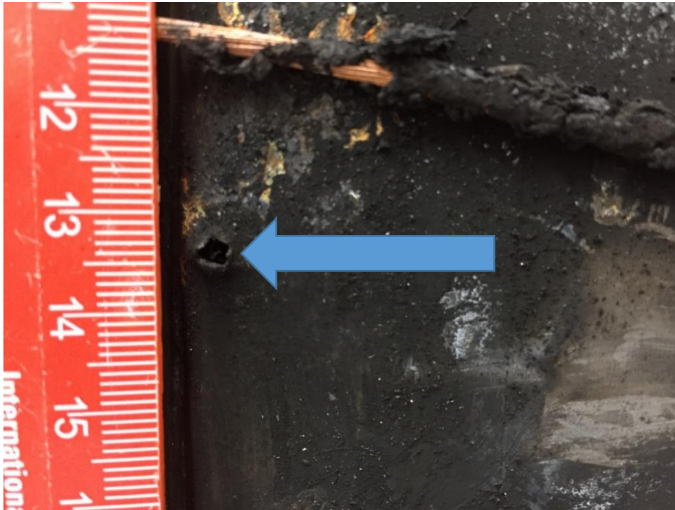
Figure S10. Photograph of the underside of the module employed in experiment 2 at the DNV GL site showing the exit hole (arrowed) of the nail.
