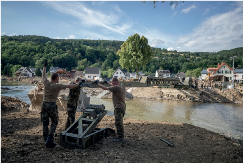
German Army pioneers erect a Medium Girder Bridge (MGB) for the residents during the flood operation in Insul in The Ahr Valley on July 26th, 2021.
