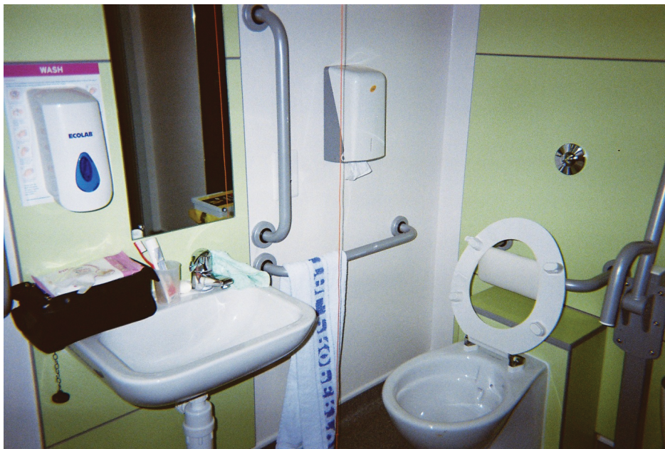
FIGURE 16 Layout of en suite where position of sink limits access to toilet. Taken by OP24, HCA, older people's ward.
