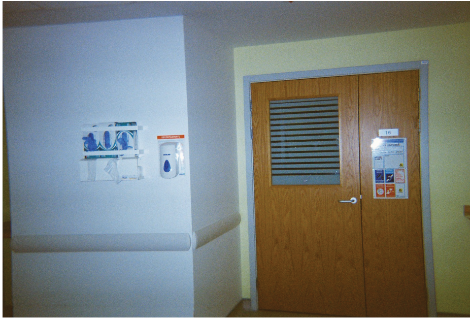
FIGURE 22 Door to a patient room, showing Vistamatic vision panel. Taken by OP24, HCA, older people's ward.
